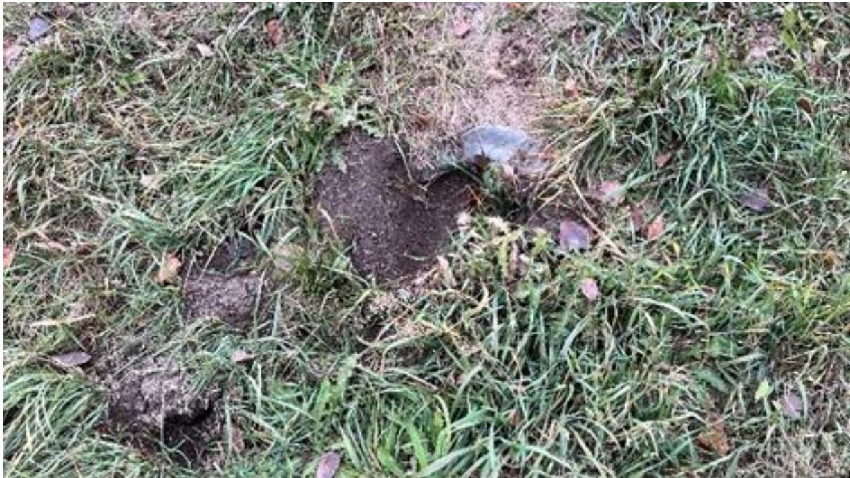
Downstream end of RR 271 culvert immediately north of Rolling Meadows Drive South
