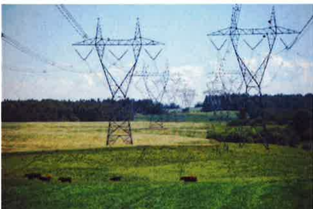
Power lines, located east of Keephills Generating Plant. Courtesy of TransAlta
