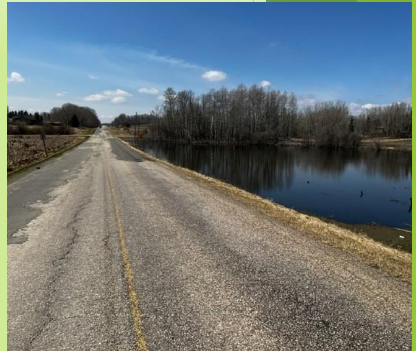
Photo: A flooded section of ditch along Mink Lake Road
